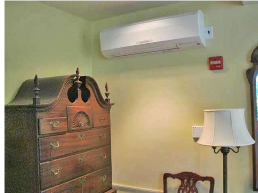
Mini-split on the wall brings heat and cold from the heat pump into the room.
